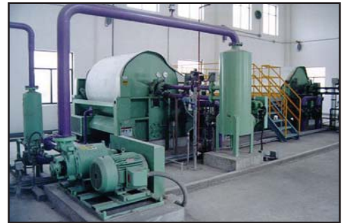
Drum Filter Vacuum System
