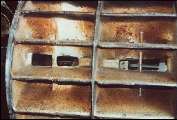
Erosion damage to rotor
