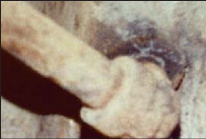
Typical Bearing Failure
